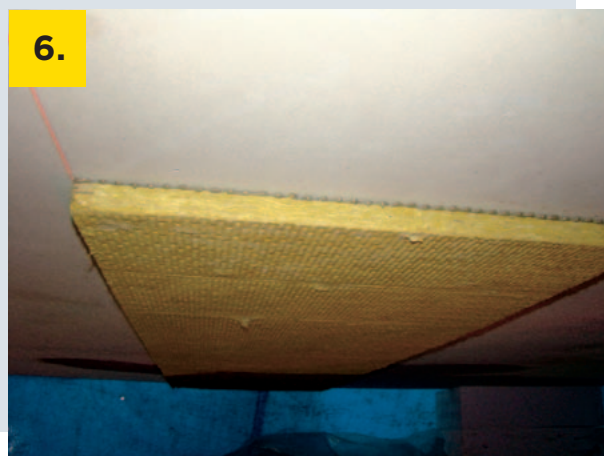
Check the bonding over the entire surface - Dexaflamm B adhesive is slightly pushed out and visible
